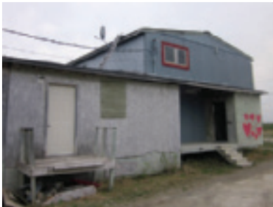
Housing for police officers. During our visit to Kashechewan First Nation, we observed that the housing for police officers needed improvements.
